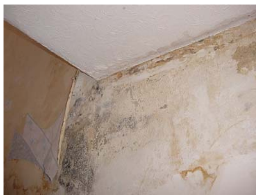
Black mould on walls as a result of severe condensation
